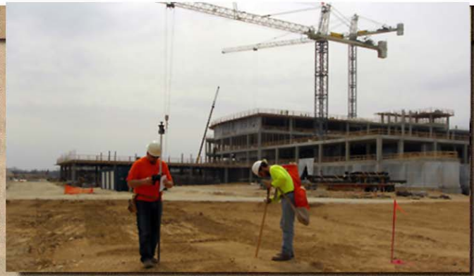
Rover units, like the one used here by R.A. Smith National's Mike Bartelson and Chad Kurtz, can be used to stake electronically, to guide manual stick-in-ground staking, and to check the accuracy of completed construction. Photo courtesy of R. A. Smith National.
