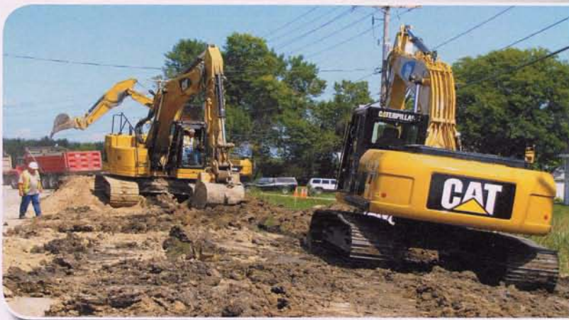
Landfill gas pipeline was installed by open cut as well as horizontal directional drilling and jack and bore.
