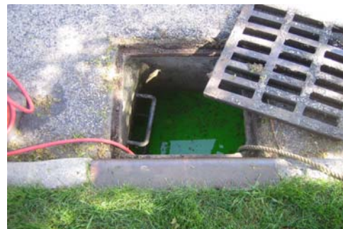
R.A. Smith National is performing dye water flooding (testing) in the City of Wauwatosa, Wis. as part of the City's efforts to evaluate the performance of their sanitary and storm sewer systems.
